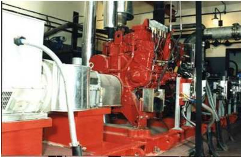
Fig. 2.2 Emergency diesel-driven pump of the system for additional emergency water supply into steam generators of Kola NPP
