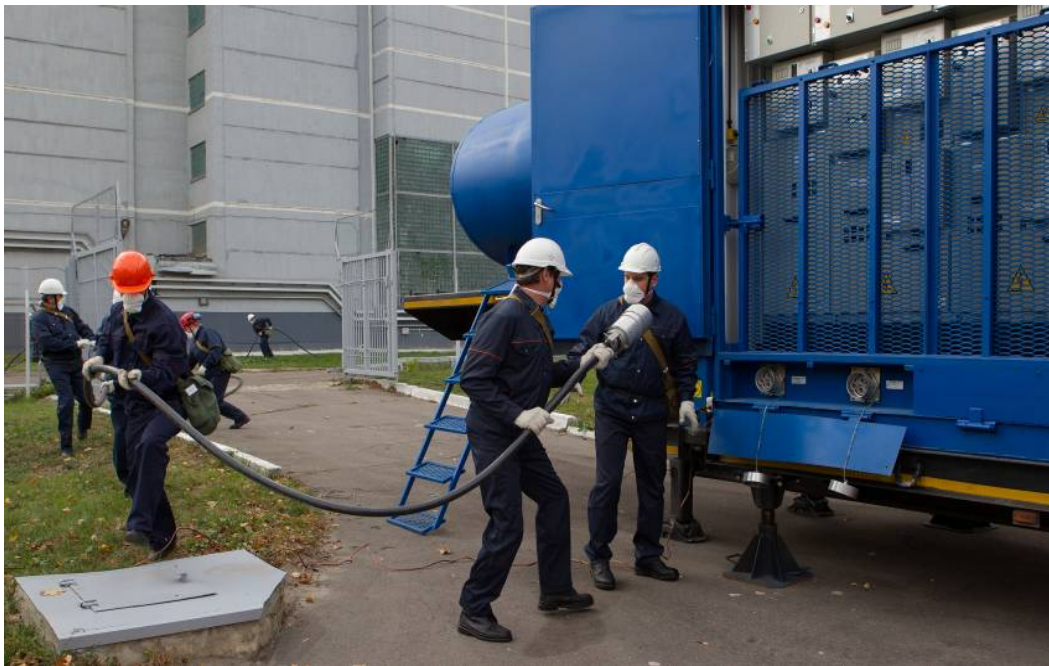
Fig. 16.5. Comprehensive emergency exercises at Leningrad NPP (2015). Training in connection of mobile diesel generator
