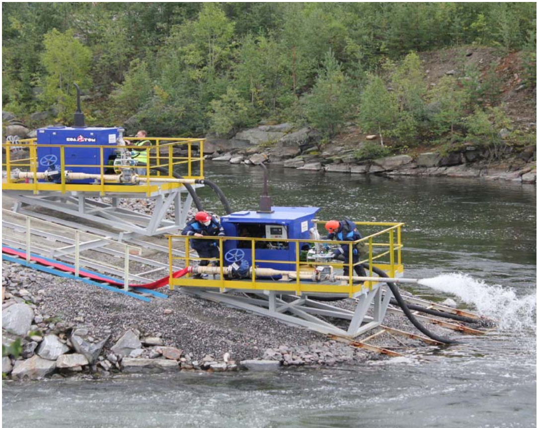
Fig. 16.7. Comprehensive emergency exercises at Kola NPP (2014). Training in connection of the pump to supply cooling water to Units 1-4 of Kola NPP
