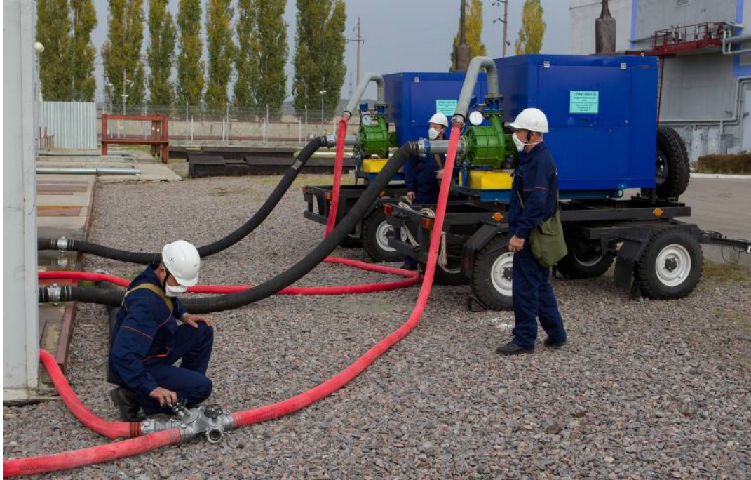
Fig. 16.4. Comprehensive emergency exercises at Leningrad NPP (2015). Training in connection of the mobile pumping unit
